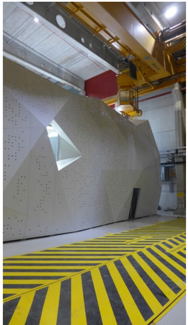
Figure 9.1. A view of LUMI datacenter (under construction) in Kone building of Renforsin Ranta business park. CSC shall be responsible for operating LUMI datacenter.
